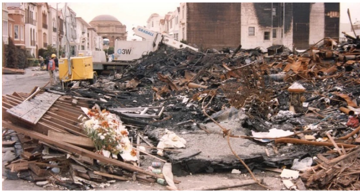
Fig. 2. Damage observed in the Eastside Tunnel post – 1989 Loma Prieta Earthquake [6]
