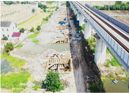
Fig. 1. Construction site plan of the new pier bearing platform adjacent to the high-speed rail line
