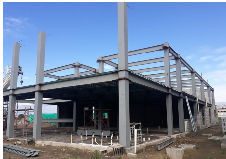
Fig. 1. Undershocked gantry of the structure under construction of the ESPE University headquarters
