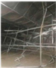
a) Reinforced tie ribs fracture
