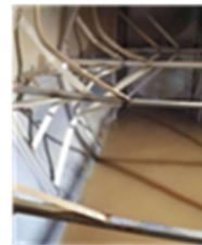
c) Reinforced tie ribs water corrosion
