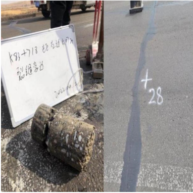
Fig. 7. Drill core sampling results of damage A
