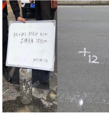
Fig. 8. Drill core sampling results of damage B
