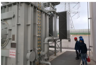
a) Power equipment
