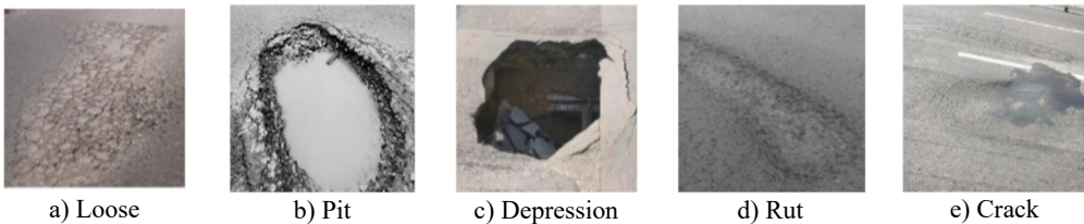
Fig. 1. Image of pavement damage types
