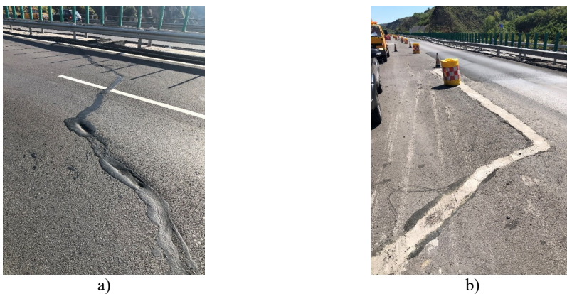
Fig. 1. The subsidence of the subgrade caused the road surface to crack
