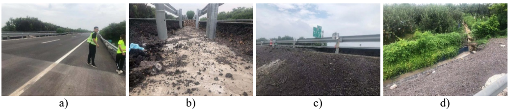
Fig. 1. Site photos of subsidence disease
