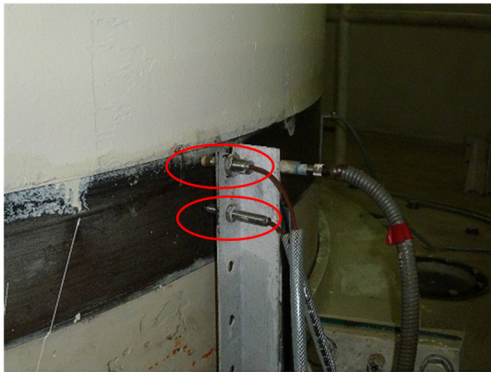
Fig. 6. Installation site of sensors
