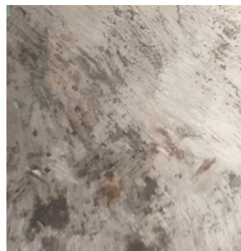
Fig. 4. The outer surface of the tube sample after the anticorrosion coating is worn off
