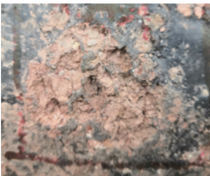
Fig. 3. The serious pipe section with “soil layer with small stone slag” is adhered to the surface
