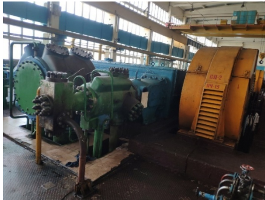
Fig. 5. General view of opposed compressor mount of in shop N4 of “KuibyshevAzot” public joint stock company
