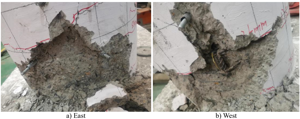
Fig. 6. The failure mode of CP
