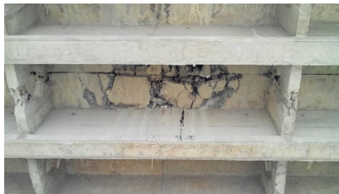
Fig. 5. Serious breakage of T beam flange in middle span of 6# span
