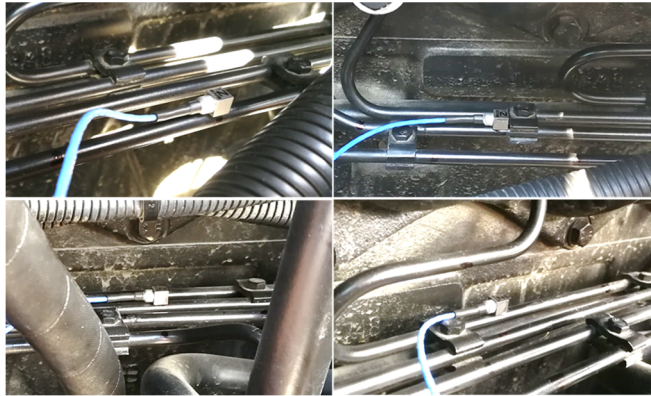
Fig. 2. Triaxial accelerometer glued on the injection pipes during measurement
