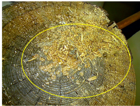
Fig. 6. Final level damage
