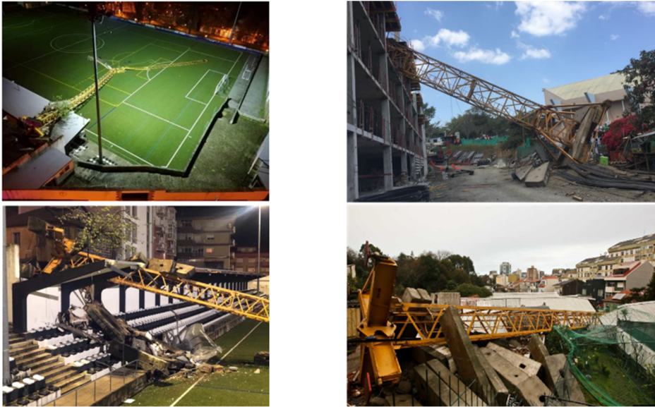
Fig. 1. Photographic register of tower crane collapses located in Portugal (left: Vila Real and right: Porto)
