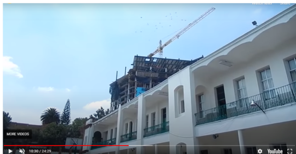
Fig. 23. Snapshot of the motion of the tower crane during the Mexico M7.1 earthquake on September 19, 2017 [22]
