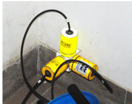
Fig. 3. Acceleration sensors mounted on the foundation of the building
