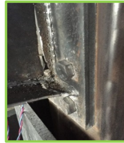
b) The cracking of the beam web
