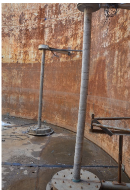
a) Overall damage result
