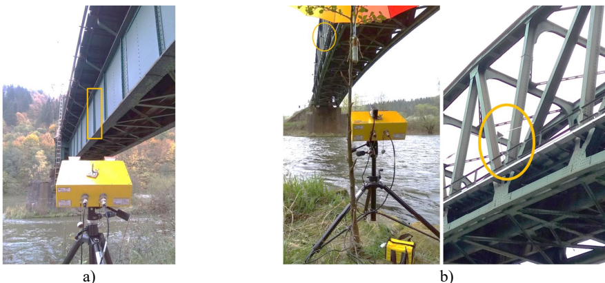
Fig. 2. Measured points: a) at box girder spans, b) at truss girder span
