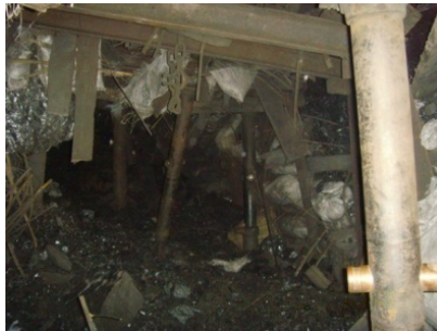
Fig. 3. The floor heave of roadway is serious
