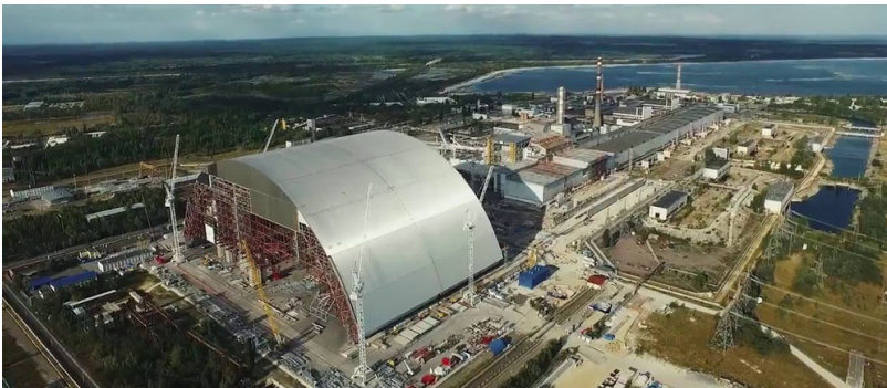
Fig. 8. The new confinement “Arka” before the sliding over the old confinement, covering the damaged structures of the fourth power unit of the Chernobyl nuclear power plant
