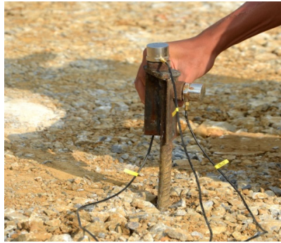
Fig. 1. Acceleration sensor installation
