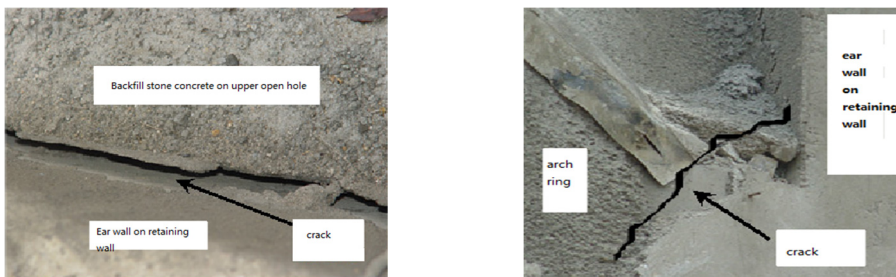
a) Retaining wall and roof backfill stripping b) Cracks at the junction of the retaining wall and arch Fig. 13. Some cracks at the exit of the right line of the Changwuling Tunnel
