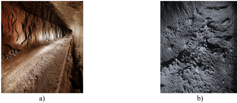
Fig. 8. Photos of a) good and b) bad condition road surface in the underground mine
