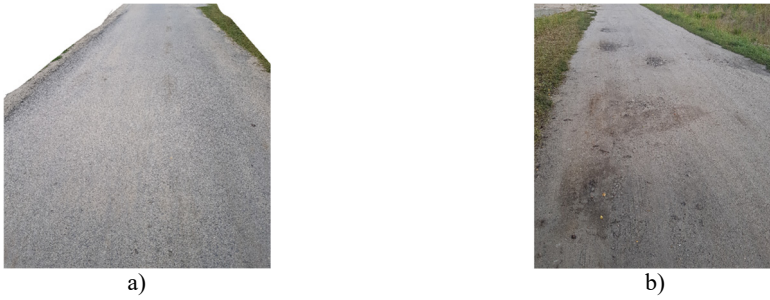
Fig. 2. Photos of a) good and b) bad condition road surface used in the test
