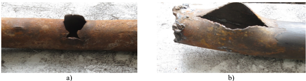
Fig. 1. Most common damage mechanisms observed in boiler water-wall with carbon steel material (Steel20): a) Surface corrosion and erosion causing wall thinning, b) thick-lip burst caused by long-term overheating and creep damage – note multiple longitudinal cracks in the vicinity of a burst
