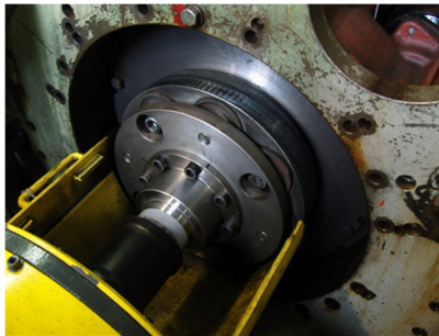
Fig. 1. Elastic coupling connecting engine and electric generator
