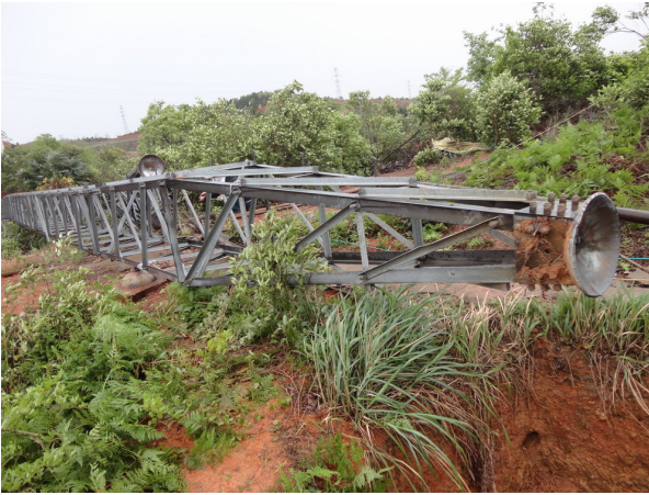
Fig. 1. The collapse accident of the #54 tower
