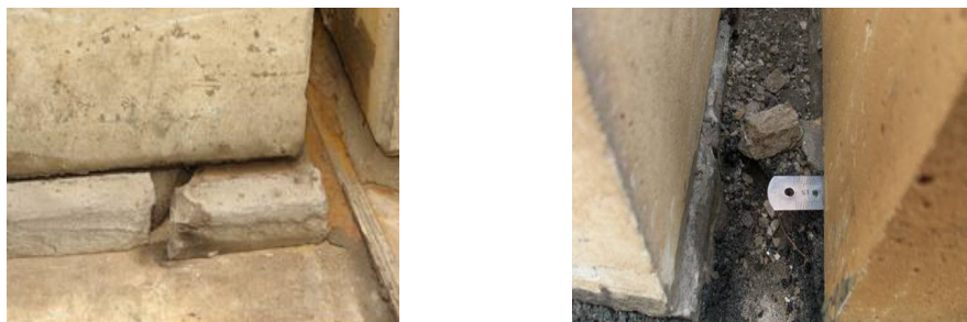
Fig. 1. Damages of ballastless tracks
