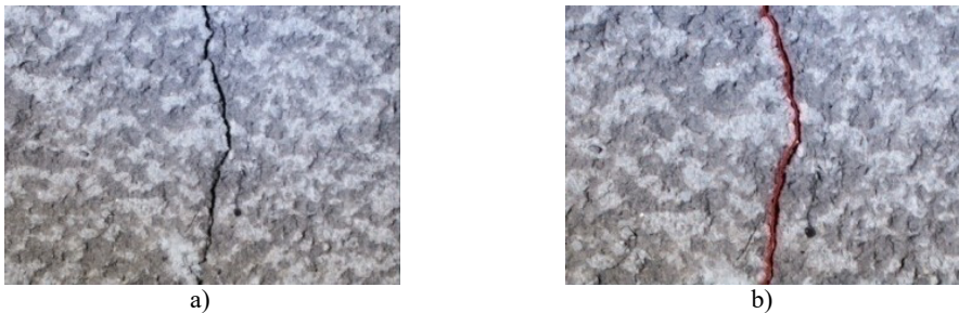
Fig. 12. Crack detection on the wall surface: a) input image, b) detected crack
