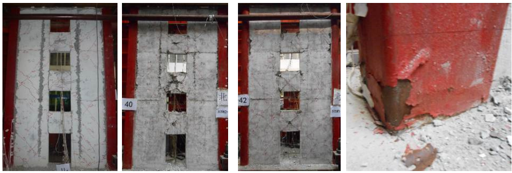
Fig. 5. Failure modes of specimens in stage I test
