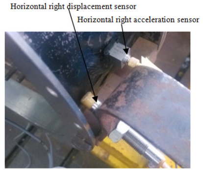
Fig. 2. Installed horizontal right of turbine casing displacement sensor and acceleration sensor local amplification
