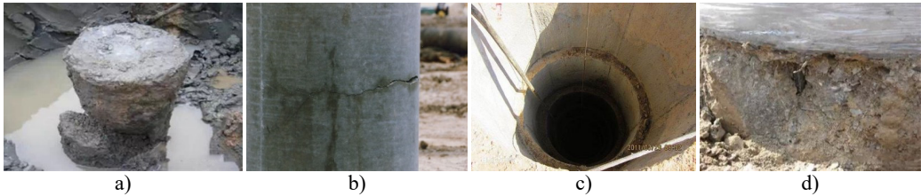
Fig. 1. The typical damage types in concrete piles: a) fractured pile, b) cracked pile, c) pile with secondary concrete pouring, d) pile with mud intrusion
