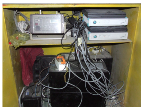
Fig. 3. A general view on developed system
