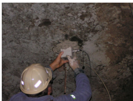
Fig. 2. Location of the sensor on the roof of the mining corridor using gypsum binder
