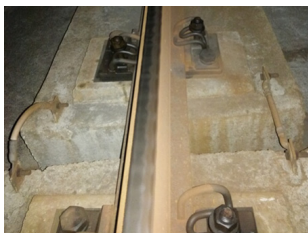
Fig. 1. Short pitch corrugation on low curved rail in Shenzhen metro line 1
