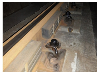
Fig. 2. Double-block non-ballasted track with the rail vibration absorbers
