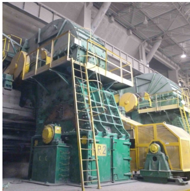
Fig. 1. A crusher – general view. Note bearings with yellow housing and location of the sensor (yellow rectangle with red dot in the center)
