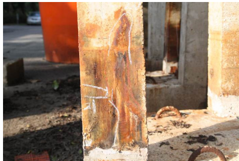
Fig. 7. Appearance of the cracks, rust and rusty spots on the surface of the specimens
