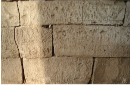
Fig. 3. Cracks in stone masonry
