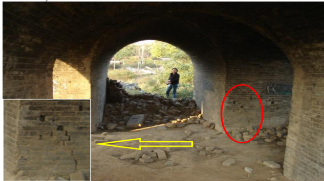
b) The distribution of the crack in the Z's direction
