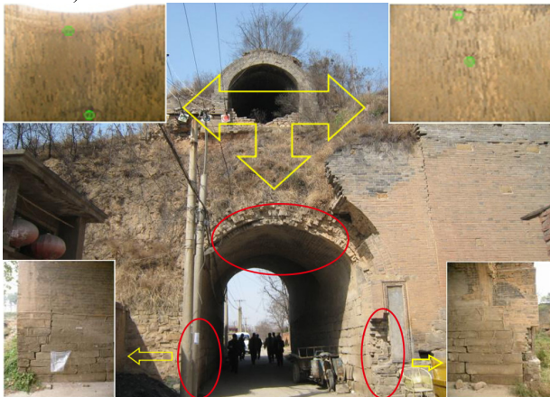
b) The distribution of the crack of the doorway
