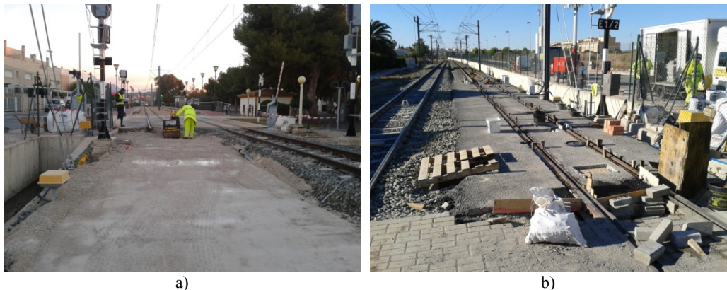
Fig. 7. a) Compaction of the graded aggregates and b) rail alignment previous to the elastomer pouring
