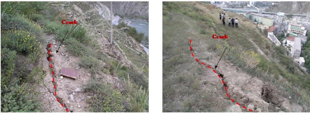
Fig. 7. Two cracks in the back scarp of the slope
