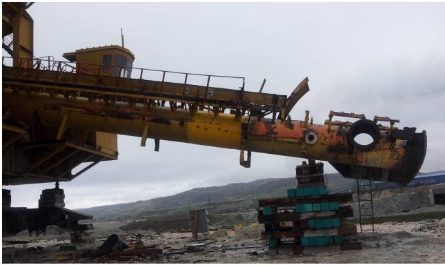
Fig. 2. BWE ER1250 bucket wheel boom with dismantled drive and bucket wheel
