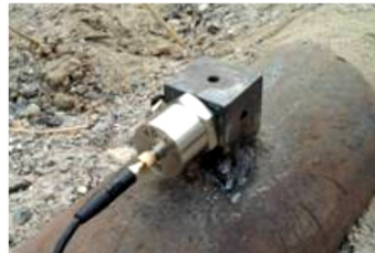
Fig. 9. Experimental installation of piezoelectric sensor
