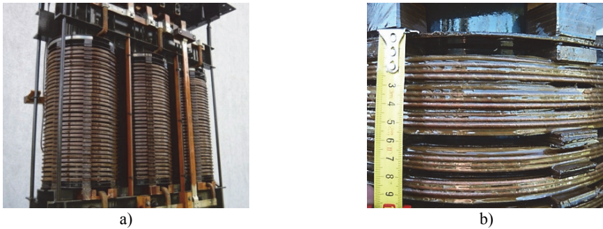
Fig. 1. a) Active part of the transformer used for the experimental tests and b) top two discs of the winding lowered
