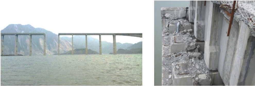
Fig. 1. Fallen girder of the Miaoziping bridge (2008 Wenchuan earthquake, China)
