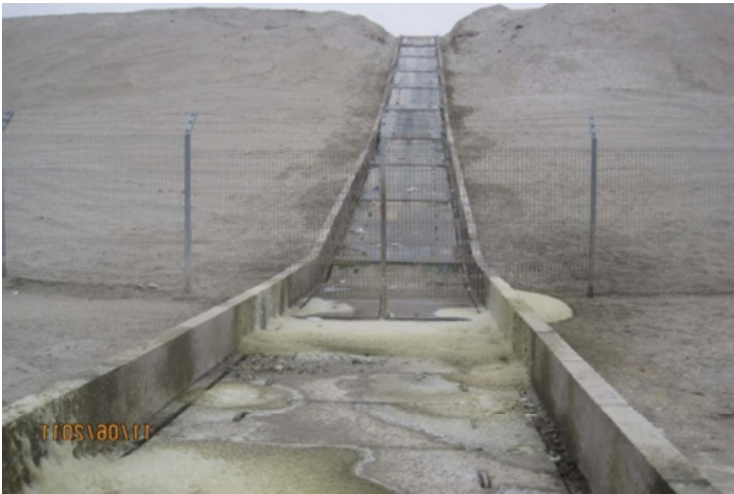
Fig. 2. Original open channel outfall at Angamos power plant
